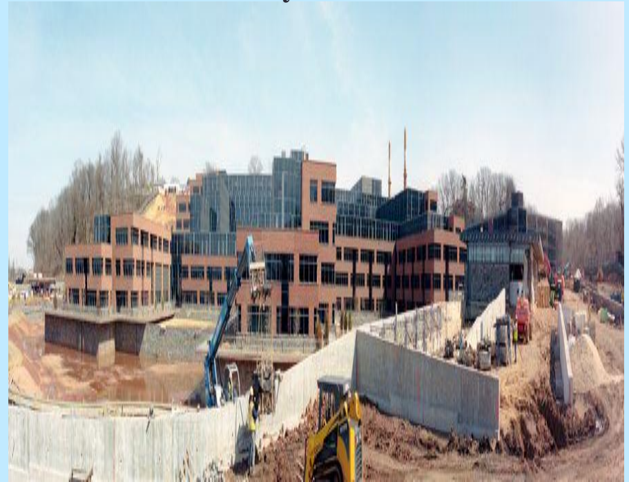
St. Elizabeth's West Campus – Central Utility Plant
